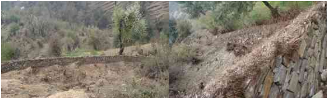
Newly constructed school compound wall, this wall is 136m long and 3f high in average
