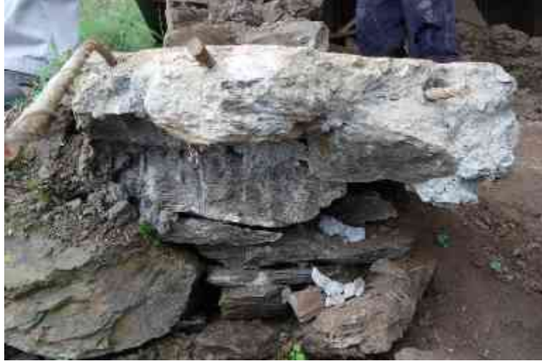
Cement Rcc made on the foundation for the stability of the office
